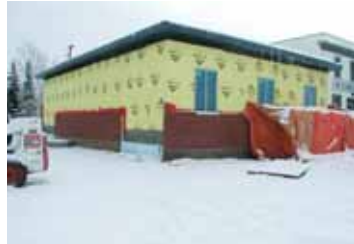
The new Edgerton branch construction in progress. Work is going on inside and out.
