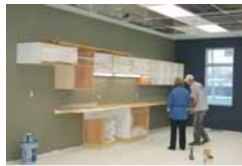
Special Projects Officer Jackie Zajic checks out the newly-installed kitchen cupboards on PlanWright's second floor.
