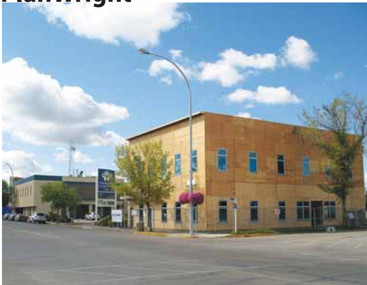
The walls are up, the roof is on, and the windows are in place at the Main St., Wainwright site. Exterior brickwork and inside electrical are well under way.
