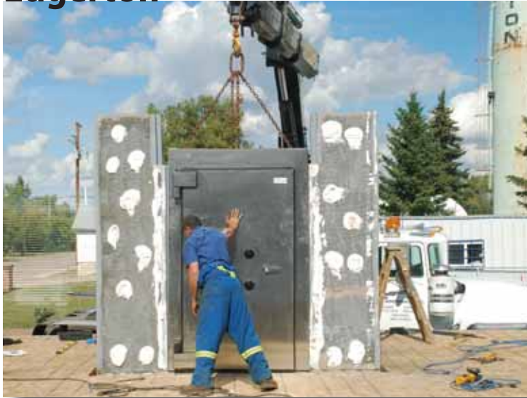
A crane sets the last piece of the vault in place at the Edgerton construction site. Next, the walls can go up around it. So that's how they do it!
